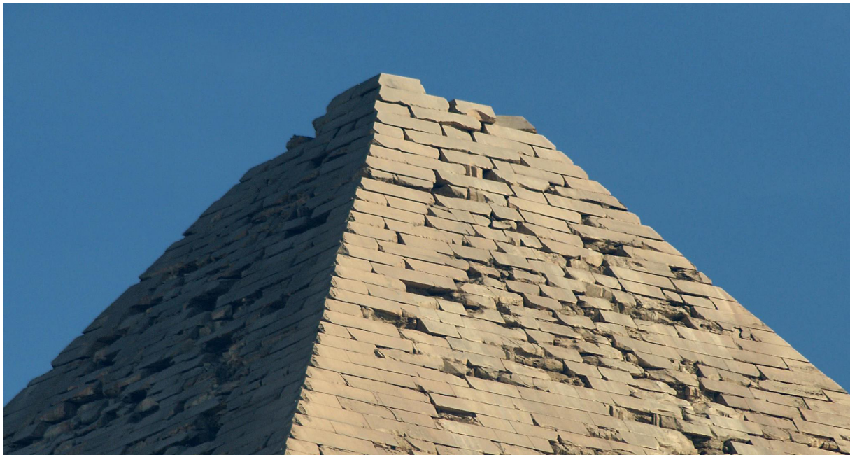
Fig. 5. Casing stones still in situ near the summit of the Pyramid of Khafre at Giza, showing a high degree of regularity which may have contributed to their structural integrity and survival. With permission © Franck Monnier.
